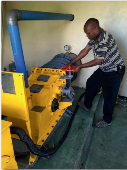
Small hydro power plant, Arusha, June 2016 (SAP no. 100261)
